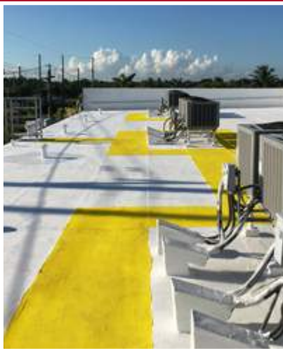
GacoFlex SF2036 WalkPad Silicone Walkway System was applied after S20 Silicone Roof Coating System.
