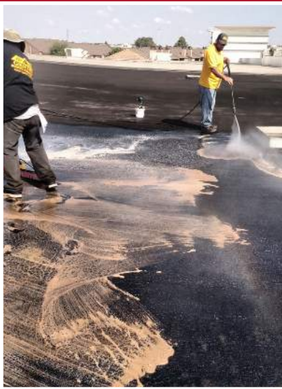
The roof was washed with GacoWash Concentrated Cleaner and allowed to dry.
